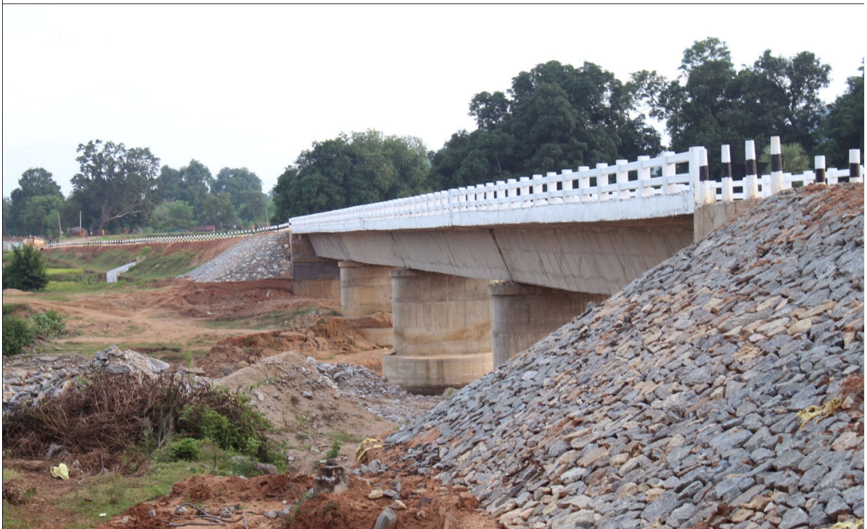
L063-PWD road to Chhatapipal road including Constriction of Bridge over Sonegarh river on PWD road to Chhatapipal ( 4 x 30.63 mtr. )under PMGSY Package No. OR-05-285/B-III.
