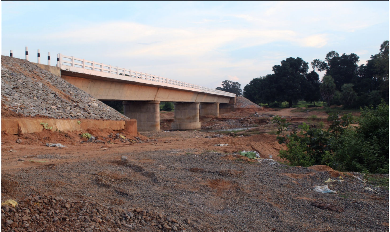
L063-PWD road to Chhatapipal road including Constriction of Bridge over Sonegarh river on PWD road to Chhatapipal ( 4 x 30.63 mtr. )under PMGSY Package No. OR-05-285/B-III.
