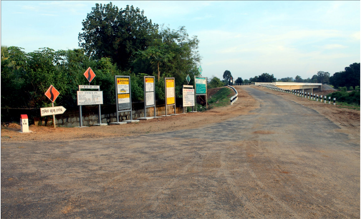
L063-PWD road to Chhatapipal road including Constriction of Bridge over Sonegarh river on PWD road to Chhatapipal ( 4 x 30.63 mtr. )under PMGSY Package No. OR-05-285/B-III.
