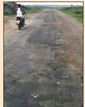
Road carriageway showing a history of routine maintenance, however now due for re-sealing / periodic renewal
