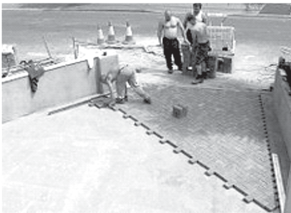
Brick paving being laid on a sand base, in south west England
