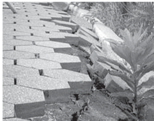
Crumbling walkway reveals details of hexagonal pavers (Base preparation & edge protection essential)
