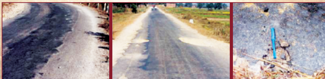
FIGURE 4. Rutting, potholes and scaling.
