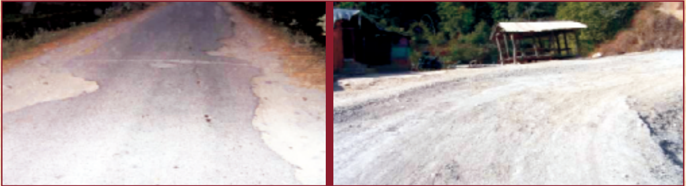
FIGURE 5. Edge breaking and raveling on curves.
